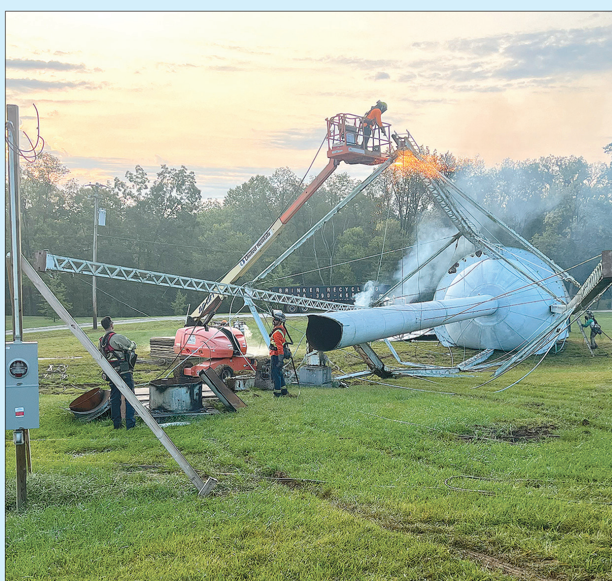
DOWN THEY COME — Crews tore down the water towers in Marthasville on Sept. 28 and Sept. 29, removing them from the city's skyline. The towers came down as part of a major improvement the city's water system. The construction of a new ground tank reservoir that is larger and higher in elevation north of Marthasville made the three tanks obsolete. The new ground tank reservoir also lowered the city's property insurance, saving the city more than $1.5 million. See more photos at warrencountyrecord.com. Photo submitted by Mayor David Lange
