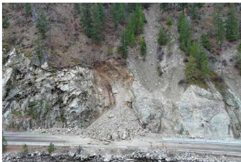
COURTESY OF WSDOT Drone pic of the slide area on South Lakeshore Road. The slide is estimated to be 1,200-1,400 cubic yards of material.
