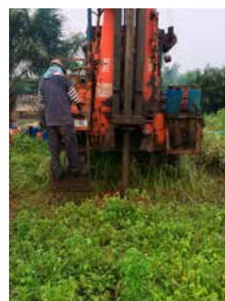
COURTESY OF IMPACT STREAM Breaking ground on an Impact Stream funded project in southern Togo that will introduce a water well, equipped with a solar pump, designed to provide reliable and clean water to a local school and the surrounding village communities that currently rely on unsanitary sources.
