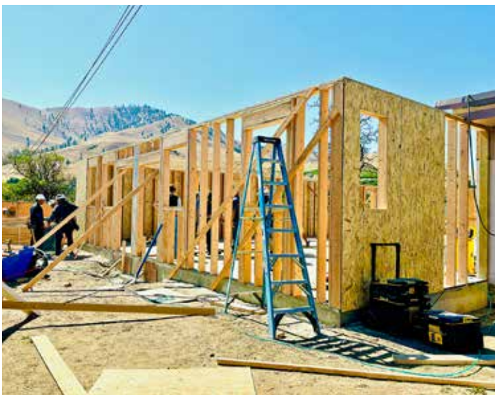
COURTESY OF LAKE CHELAN FOOD BANK Construction is on schedule to be finished by spring of 2025. SEE STORY PAGE 19
