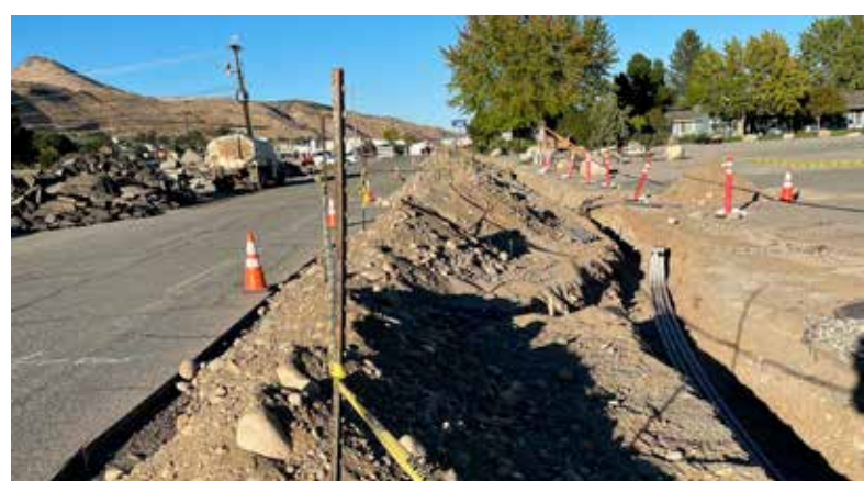
MIKE MALTAIS/WARD MEDIA Commercial Avenue looking east. The excavation will allow electrical and other infrastructure upgrades to be installed.
