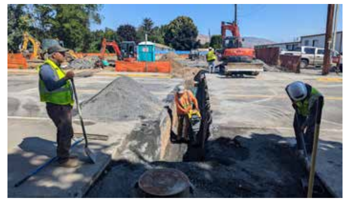
COURTESY OF COMMON GROUND COMMUNITY HOUSING TRUST Construction workers install upgraded sewer connections for the Craik Cottages affordable housing project in Wenatchee. The project, managed by Common Ground Community Housing Trust, received funding from Chelan County's Cascade Public Infrastructure Fund to support the completion of eight cottage homes for low to moderate-income households.
