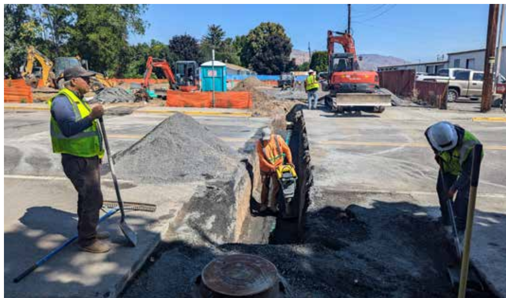
COURTESY OF COMMON GROUND COMMUNITY HOUSING TRUST Construction workers install upgraded sewer connections for the Crail Cottages affordable housing project in Wenatchee. The project, managed by Common Ground Community Housing Trust, received funding from Chelan County's Cascade Public Infrastructure Fund to support the completion of eight cottage homes for low to moderate-income households.
