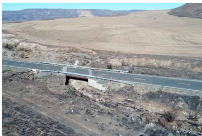
COURTESY OF DOUGLAS COUNTY TRANSPORTATION DEPARTMENT An aerial image of the Upper Pearl Hill Bridge shortly after the Cold Springs Canyon/Pearl Hill Fire on September 7, 2020. The bridge experienced significant structural damage and is being replaced.
