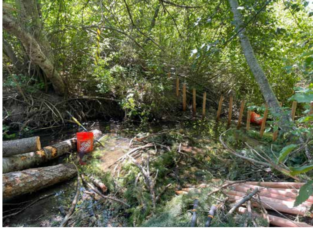
The work team added large wood and a beaver dam analog (BDA) in a segment of Chumstick Creek. This slows water flow, which provides a number of different ecological benefits.
