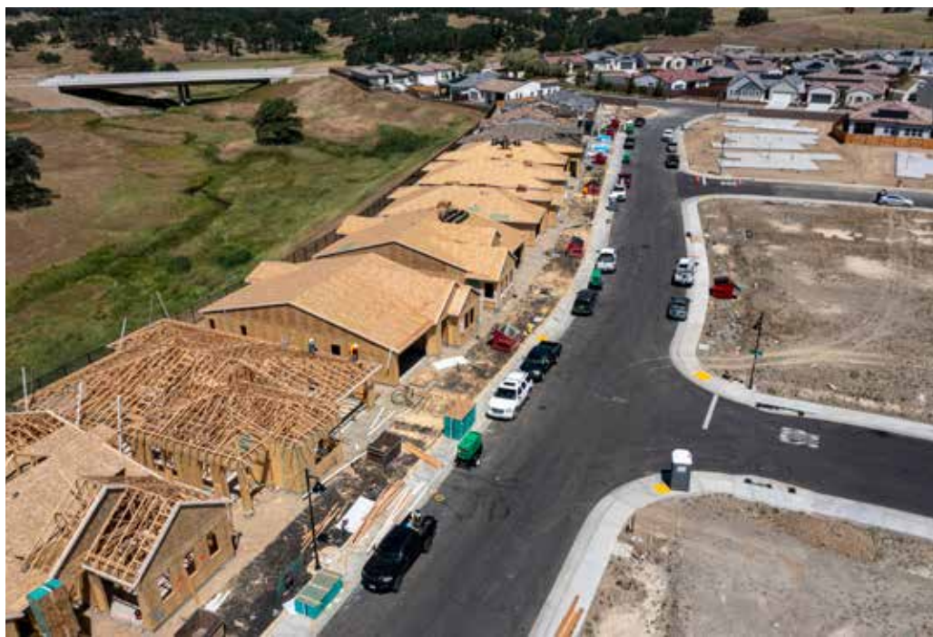
Houses under construction at the Toll Brothers Regency at Folsom Ranch community in Folsom, Calif., on Thursday, May 18, 2023.
