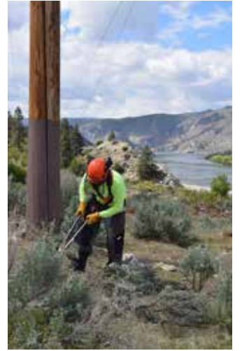
COURTESY OF CHELAN PUD A contract worker clears brush around a transmission structure in Chelan County.
