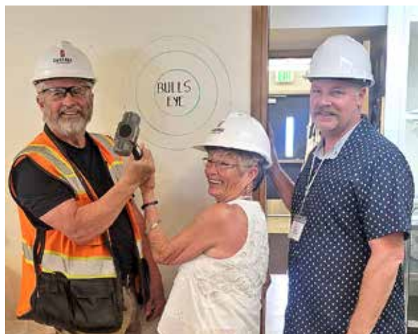
RUTHEDNA KEYS/WARD MEDIA Timi Starkweather, former Heritage Heights Board Chair, is shown with Christian Hansen (left) and Mike Campeau (right) of the CareAge Construction crew who has started construction of the Memory Care Unit, End-of-Life Suites and kitchen remodel, and other upgrades at Heritage Heights.
