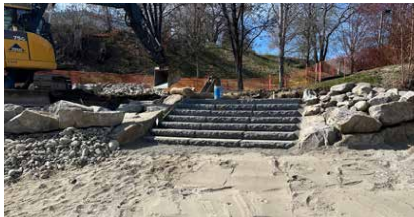
The Riverwalk Park project is on-time and going well. Pipkin crews are finishing the flat-rock staircase for the waterfront access point at site A, between W. Okanogan Ave. and W. Woodin Ave. Crews also installed split-rail fencing at site B, near the wooden viewing area, to help protect newly rehabilitated shoreline from further erosion, encourage native plantings to establish, and encourage visitors to use the improved waterfront access points when they're finished. Next, crews will work on landscaping, and then paving the trail by late April, pending weather.
