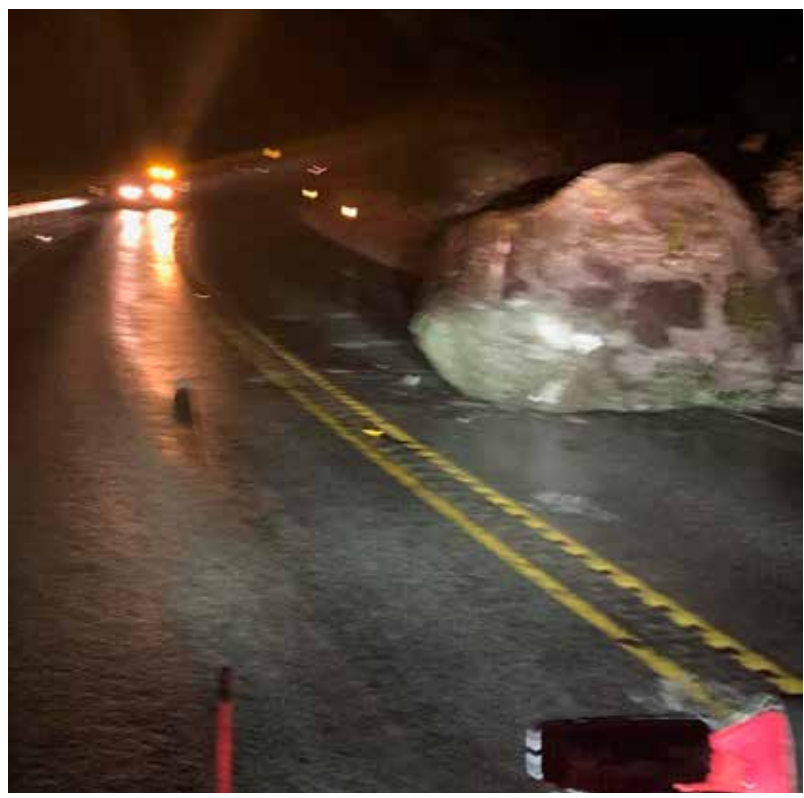
A massive boulder, about the size of a car, blocks a traffic lane on Highway 2 in Tumwater Canyon near Leavenworth, discovered early on Feb. 6 by a Washington State Department of Transportation crew during a routine check. The imposing rockfall prompted a controlled explosion to ensure the safety and passage of motorists in the area.
