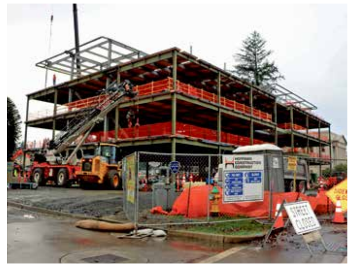
ASPEN ANDERSON / WASHINGTON STATE JOURNAL The Newhouse building is currently under construction as part of the Legislative Campus Modernization for its replacement.
