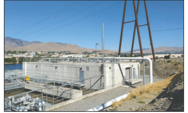
New 2nd Generation ATAD Reactors
