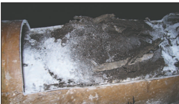
Fouled Jet Aeration Header
