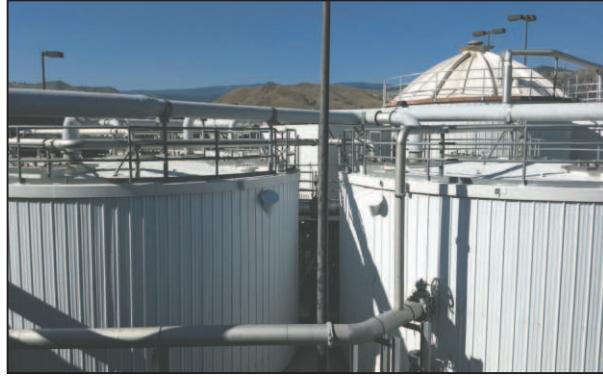
1st Generation ATAD Reactors converted to SNDRs
