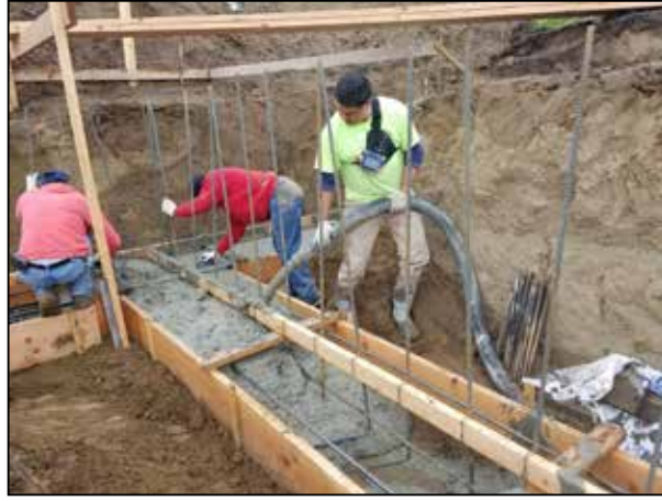
Left is Obed's younger brother Bernardo, who operates one of the concrete line pumps. Bernardo Maravilla (on right) is business partner and pump operator Samuel Gallegos.
