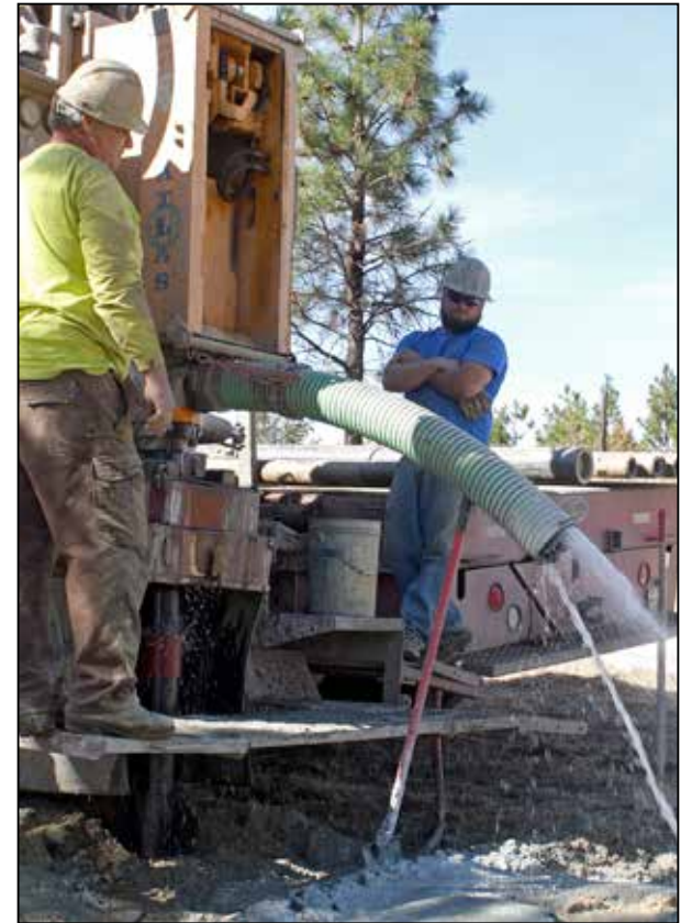
Tumwater workers monitor the flow of water.
