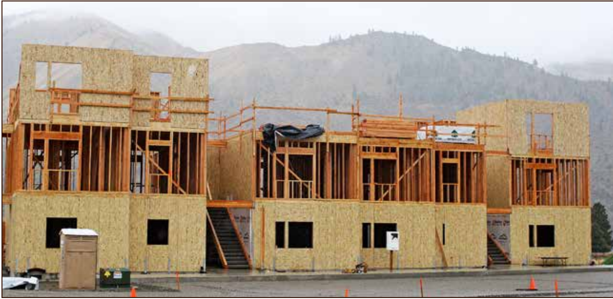
This framed building will eventually be home to the 12-unit Entiaqua Apartments, ready for occupancy June 2020.
