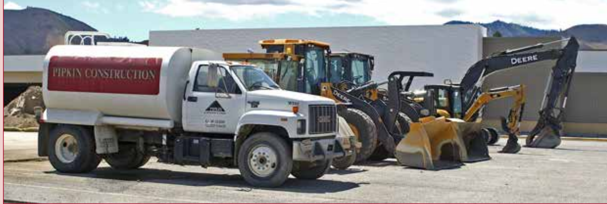
The sign is up and heavy equipment stands at the ready to make millions of dollars in improvements to the inside and outside of the former Shopko building across Maple Street from the Postal Service on North Wenatchee Avenue.
