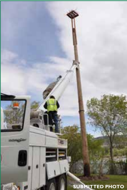
SUBMITTED PHOTO PUD power pole in the Appleyard, just south of Wenatchee.
