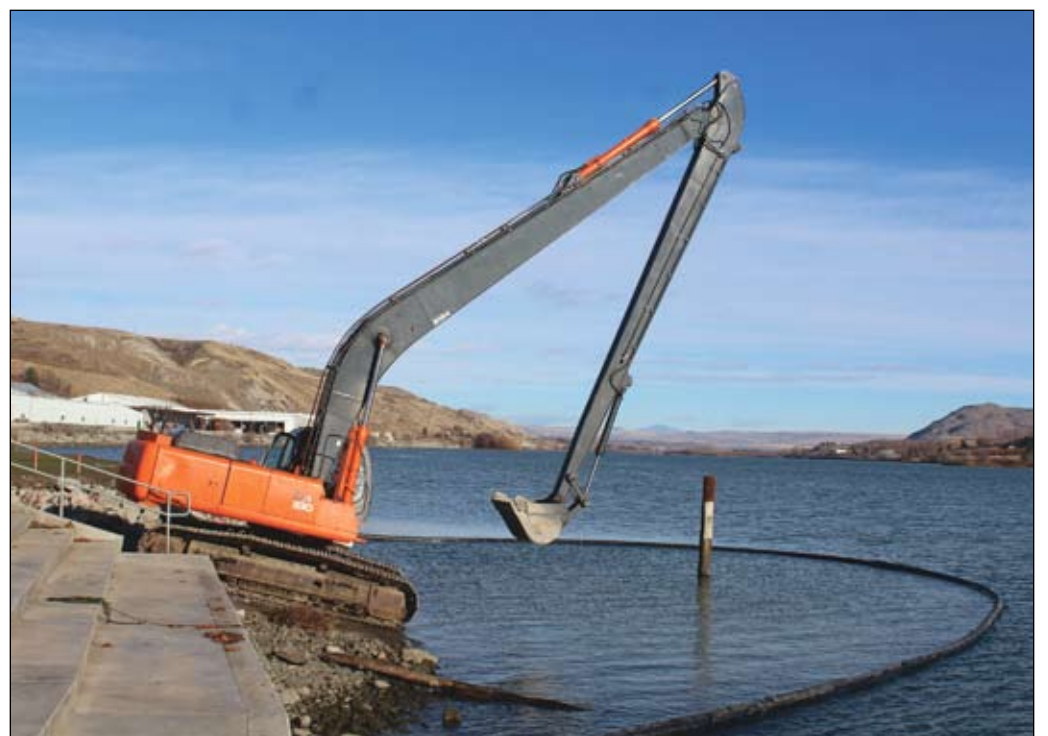
Photo by Mike Maltais The Douglas County PUD is busy at Ives Landing and along Memorial Park, replacing docks and upgrading the bulkhead and access points for recreationists.
