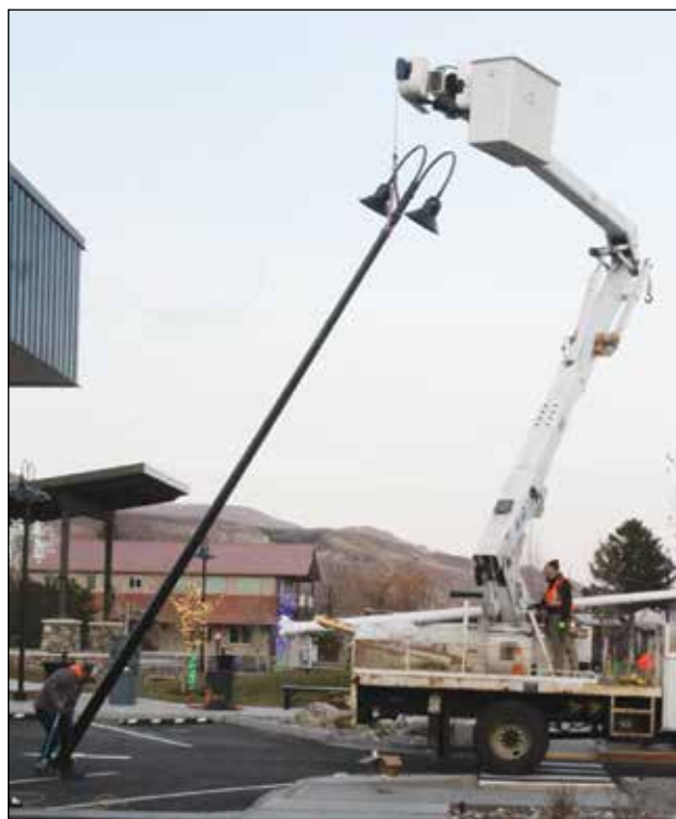
Workmen installed one of the final lamp posts near the pump station last December.
