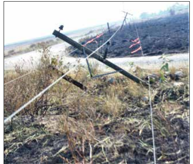
Downed power lines on Cameron Lake Road are tagged to warn approaching drivers of the danger.
