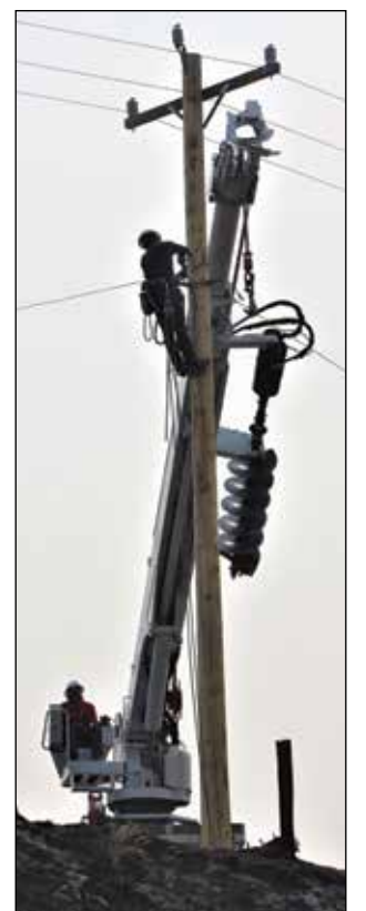
A Douglas PUD worker mans the auger and hoist as a lineman guides a line into place on a new pole installed along Road B N.E. between Bridgeport and Mansfield.
