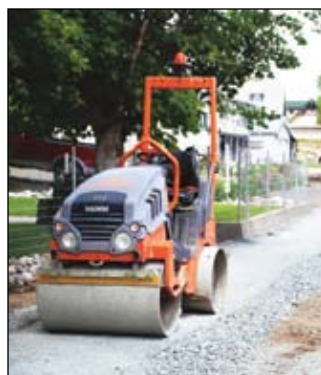
Construction work is underway to install a sidewalk along the north side of Warren Avenue from Riverside Drive east to about Chris Street.
