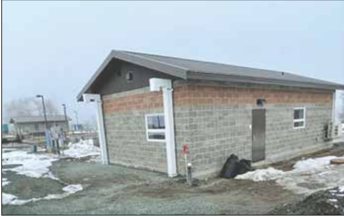
The rebuilt Bridgeport wastewater treatment lab was scheduled to be occupied and operating by the end of January.
