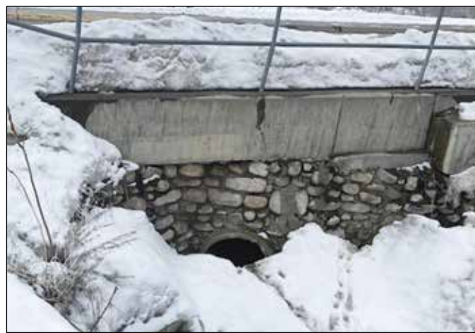
This culvert near the intersection of Seventh Street and Paradise Hill Road would be replaced with a larger one as part of the part of Brewster’s proposed flood control measures.
