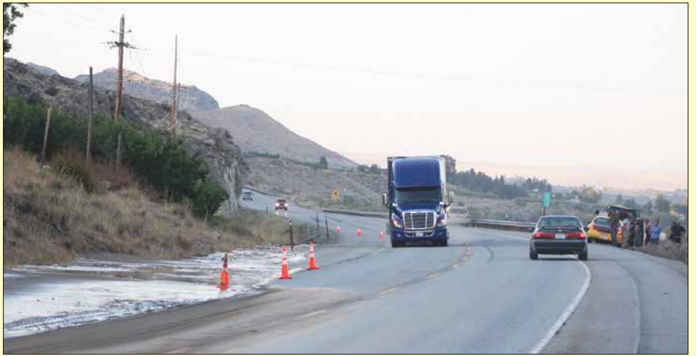
Westbound traffic on Highway 97 was diverted between Pateros and Brewster last Friday evening, July 14 as a crew responded to excess water and a minor mudslide encroaching onto the roadway. Mike Maltais/QCH
