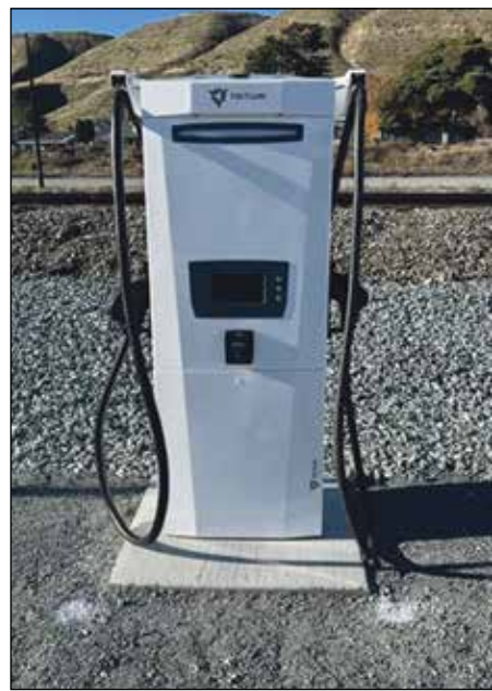
This level two charger is one of three types at the Pateros station.
