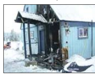
Photo courtesy of CF&R#7. Damage was limited to the utility room and is considered re-buildable at a home in Union Valley that was damaged by fire on Dec. 16.
