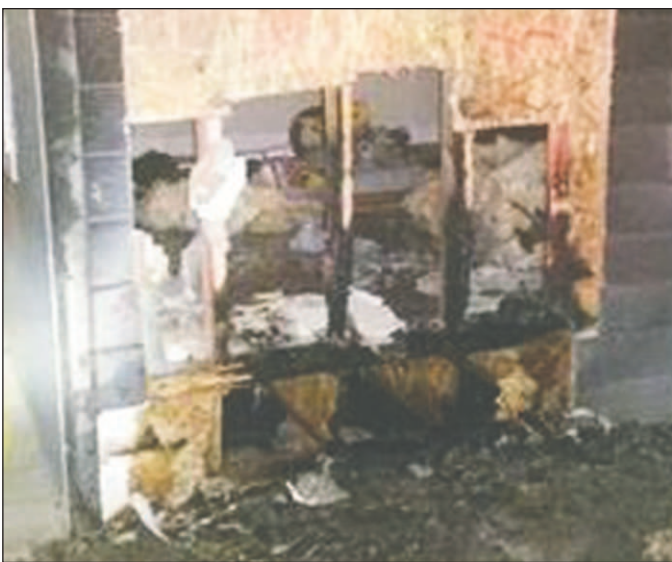
Photos courtesy of Chelan Fire and Rescue Flames burned through an exterior wall and damaged part of the new home's front room.
