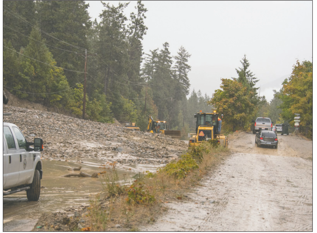
LEFT: County crews looks at the rocks and mud in the catch basin. ABOVE: Those living on the south shore were able to use a bypass road until the main road was cleared.
