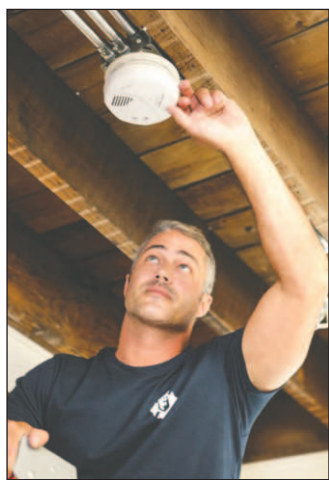
BPT Testing and maintaining alarms is key. Alarms should be tested regularly and replaced at least every 10 years.
