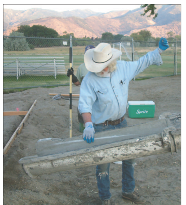
ABOVE: Volunteer Randy Doull guides the first pour of concrete for the new playground equipment at Singleton Park. LEFT: Architect drawing of new playground equipment for Singleton Park.
