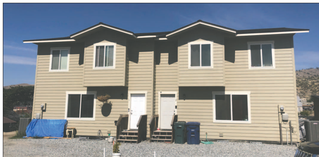
KATIE LINDERT/WARD MEDIA Lake Chelan Valley Habitat for Humanity is constructing eight homes for eligible community members. This new development, known as Pumpkin Lane, is a cul-de-sac addition located in the 600 block of Wapato Avenue.
