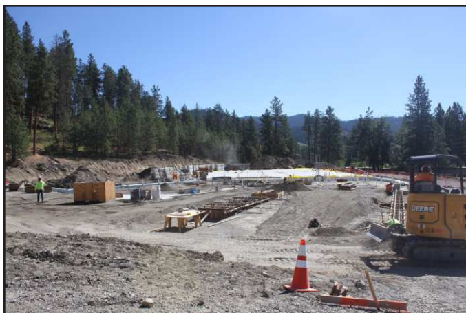
This is a view of the high school construction. Everything is currently proceeding on schedule. Excavators did find some bad material underground initially, which had to be removed.
