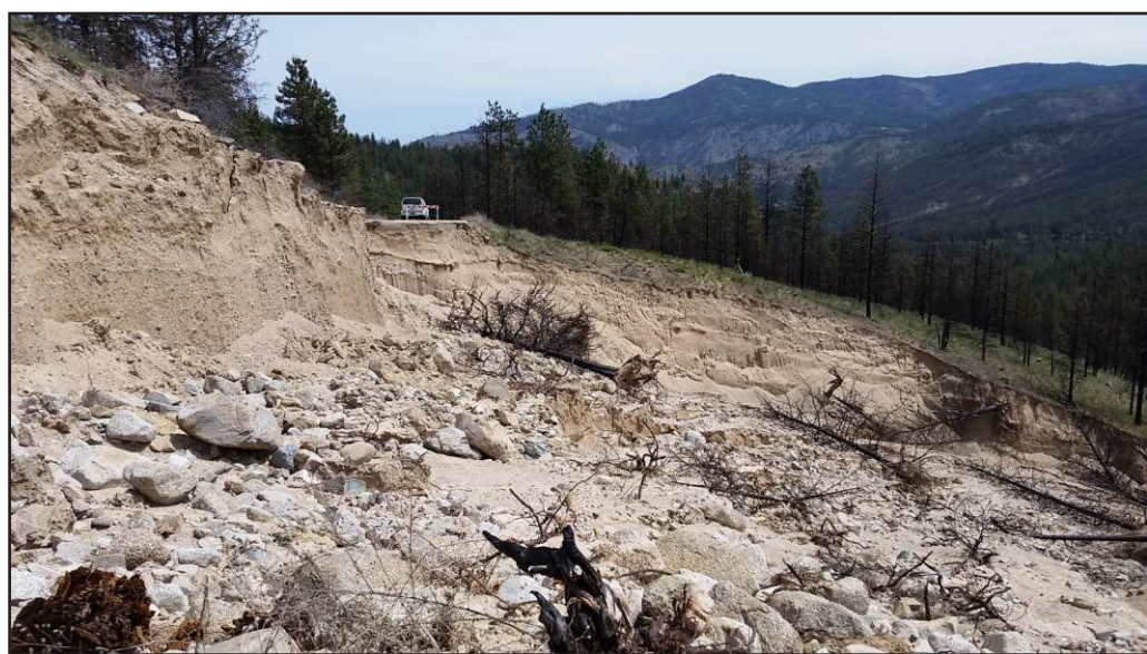
Photo submitted by Molly Williams and D. Colbert The Black Canyon Road, #4010, near Winthrop, WA sustained extensive road damage from 2016 flooding. The Cougar Creek Road #5008-200 washed out during spring rains in April 2016.
