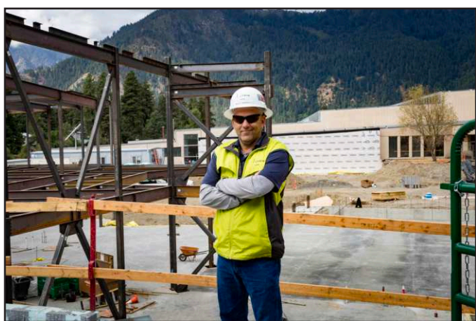
Photo submitted by Marlene Farrell Barry Meredith, Lydig superintendent, stands on the 2nd floor of the new Cascade High School construction.
