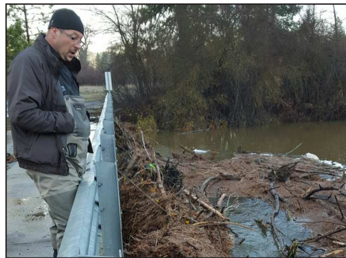
File photo Debris from the the 2015 flood piled up against the bridge at the hatchery.
