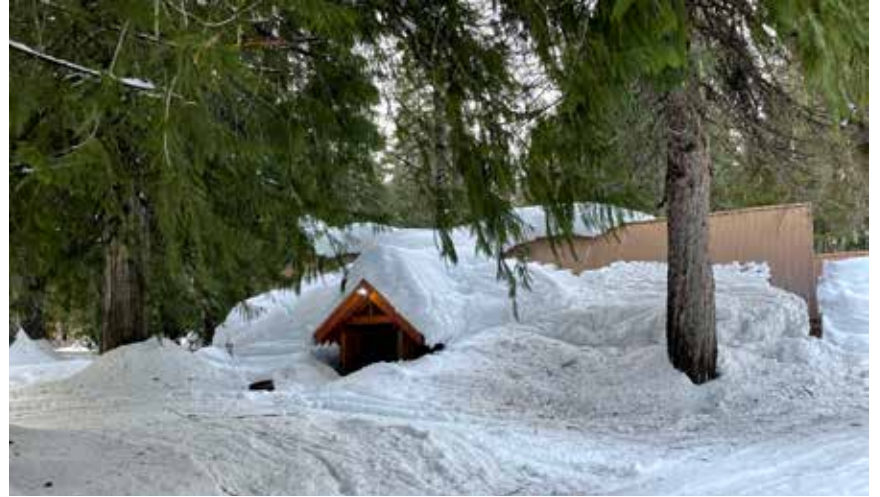
PHOTO SUBMITTED BY ZACHARY MILLER. Tall Timber staff and volunteer housing unit engulfed in snow.
