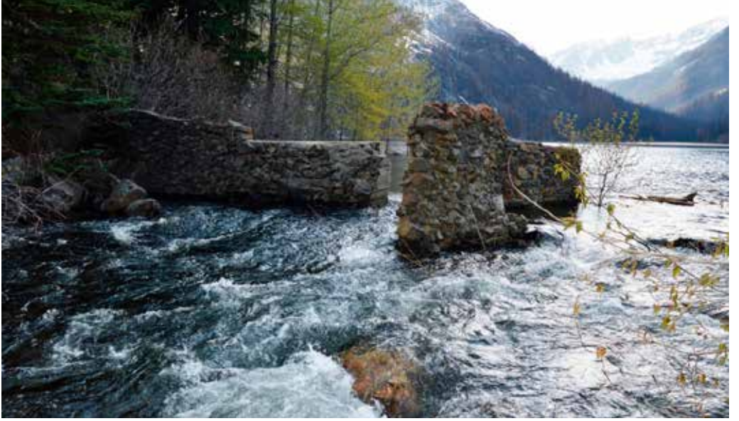
In the spring of 2018, floodwaters, and runoff overtopped Eightmile Dam.
