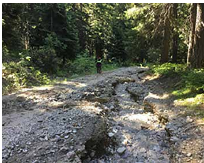
PHOTO CREDIT: USDA FOREST SERVICE PHOTO BY KEN BIGELOW, FOREST SERVICE CIVIL ENGINEER. Rock and mud debris and rutting damage on the #6200 road above Dry Creek Bridge, June 2023.
