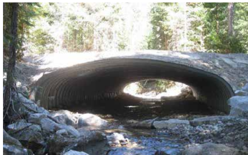
PHOTO BY MCLAIN JOHNSON, WENATCHEE RIVER RANGER DISTRICT FISHERIES BIOLOGIST, USDA FOREST SERVICE. This is an example of one of the newer style of bottomless arch culverts that allows fish and other aquatic organisms passage under a road. This one is located along the Alder Creek Road #6208 on the Wenatchee River Ranger District.
