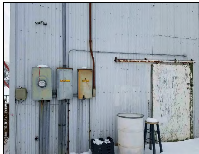
This the back view of the press box that FMHS is looking for funding to replace. Demolition could begin over spring break.
