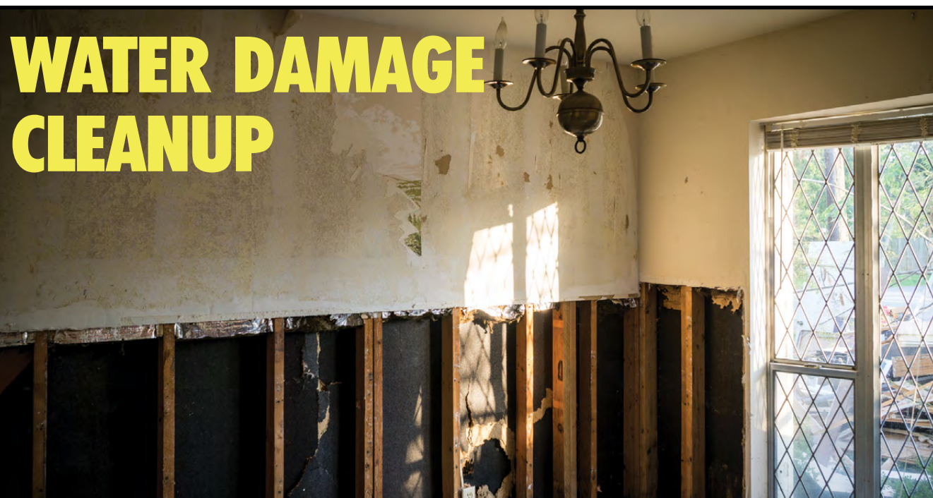
Whether the source is a natural flood or a broken pipe, excess water in a building can leave severe amounts of damage, both immediately and in the long term. To prevent your home or business from losing value and to protect your belongings, rapid emergency mitigation is an important service to call upon.
