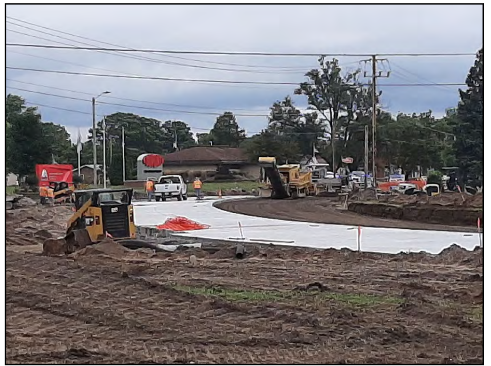
Workers with Jones Contracting out of West Point work on the southside lane of Avenue L in August. Concrete has already been poured on the north bound lane. The city took some of the curve out of the stretch of Old Hwy. 61. Data showed the segment was one of the higher rated accident zones on the stretch of roadway.
