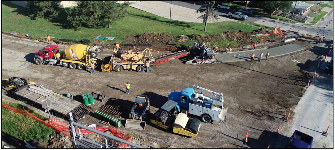
This section of Hwy. 61 that was poured on June 11, had to be torn out due to a design error, the cost of which was absorbed by the engineering firm on the project.
