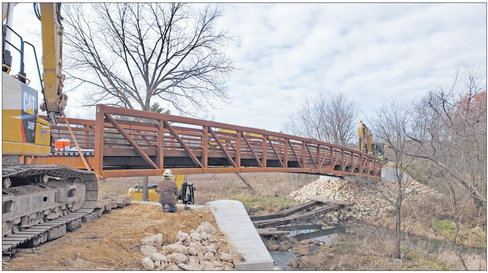
Workers move a new bridge into place on the Elroy-Sparta State Bicycle Trail east of Kendall. The bridge is one of two that had to be replaced after the flood of 2018 damaged sections of the trail. Contributed photo
