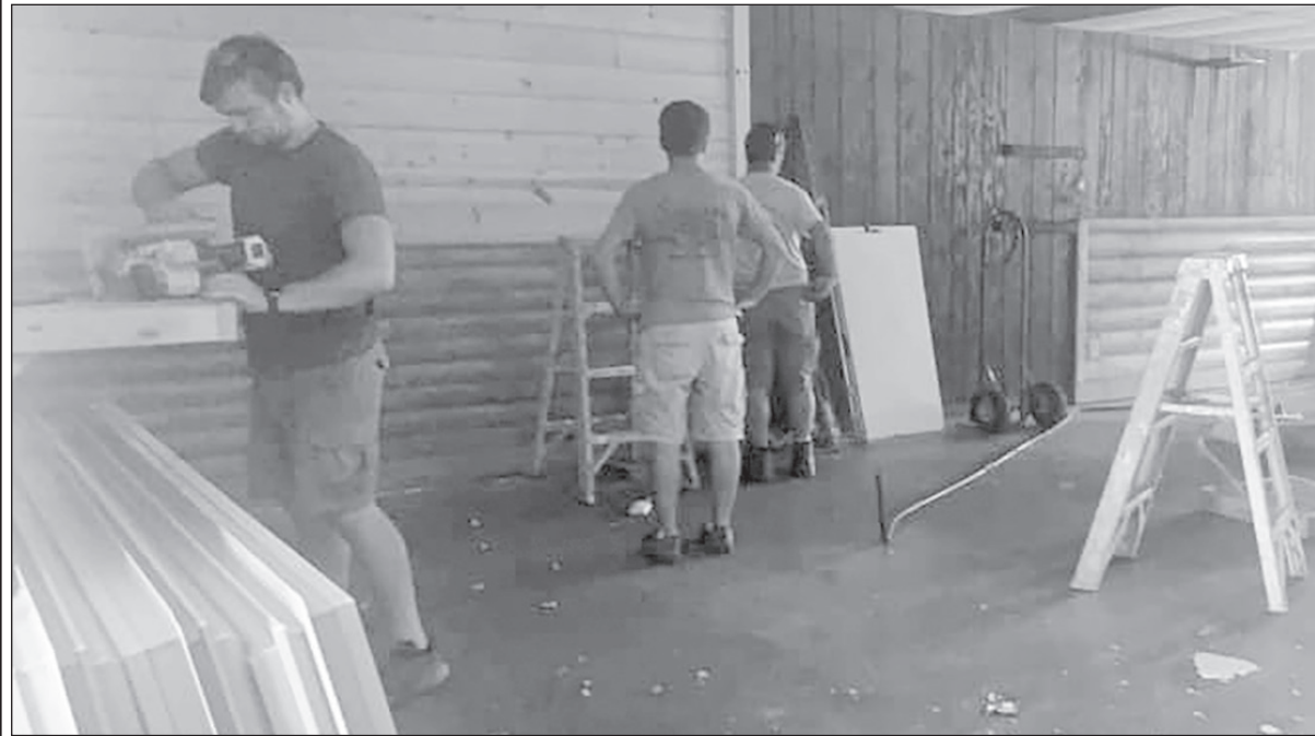
Efforts to remodel the former Misfit Tap into a childcare facility have been ongoing since June, and owner Jenni Schrock hopes to have the facility ready for a September 1 opening. Contributed photo.
