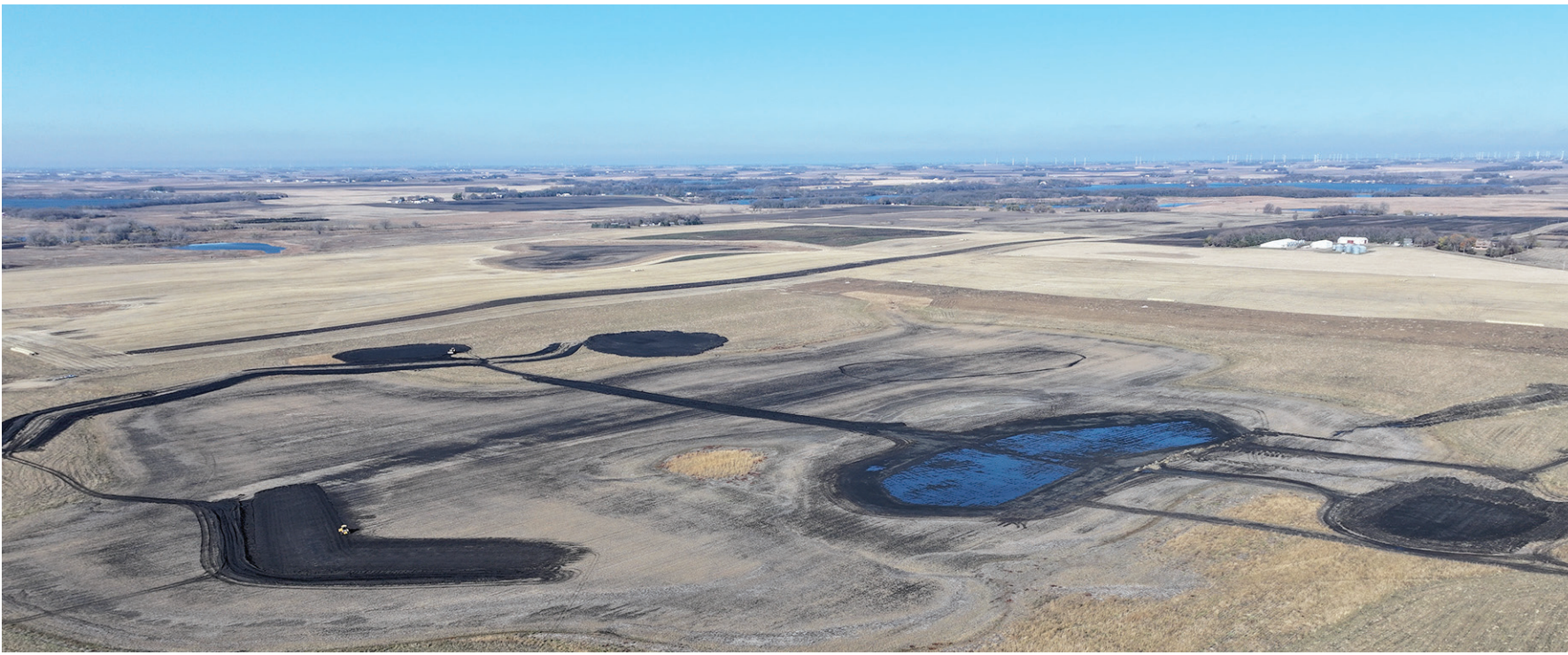
Landscape photo of early stages of wetland restoration work facing NW. Sediment removal can be seen already holding water and some tile removal lines are also visible, as well as embankment construction restoring the natural shoreline.
