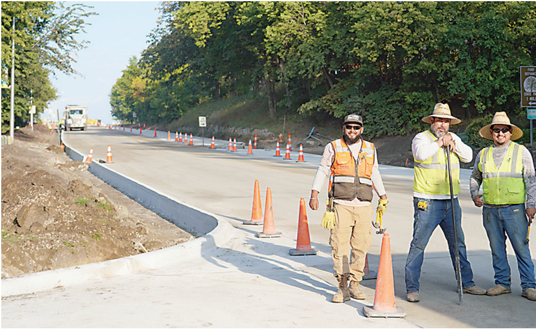
Road crews have been busy paving the rest of Highway 9 West this past week. Area residents anxiously await when they can use the busy highway as normal.
