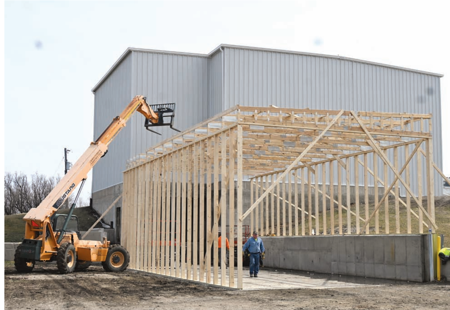
TRANSFER STATION BUILDING PROGRESS - Work on the new Transfer Station continues. The new bay for trailers was framed at the end of last week. The ground to the left shows the imprint of the previous bay. -Drew Hansen photo
