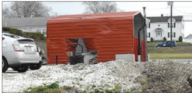
The Wing-N-It restaurant smokehouse was left with a gaping hole after a drag race car crashed through it Thursday, April 10.
